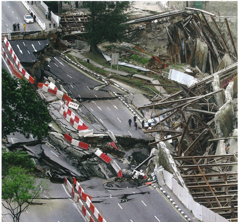
Above: The Nicoll Highway collapse of 2004
