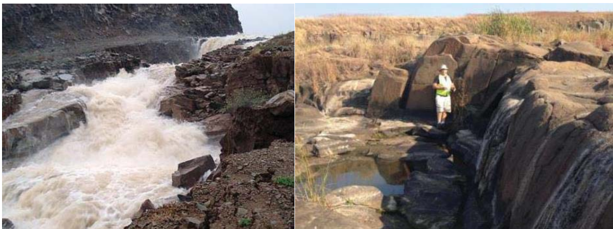
Figure 4. Erosion of blast-damaged rock at Osplaas dam (left) and weathered dolerite at Klipfontein dam (right)
