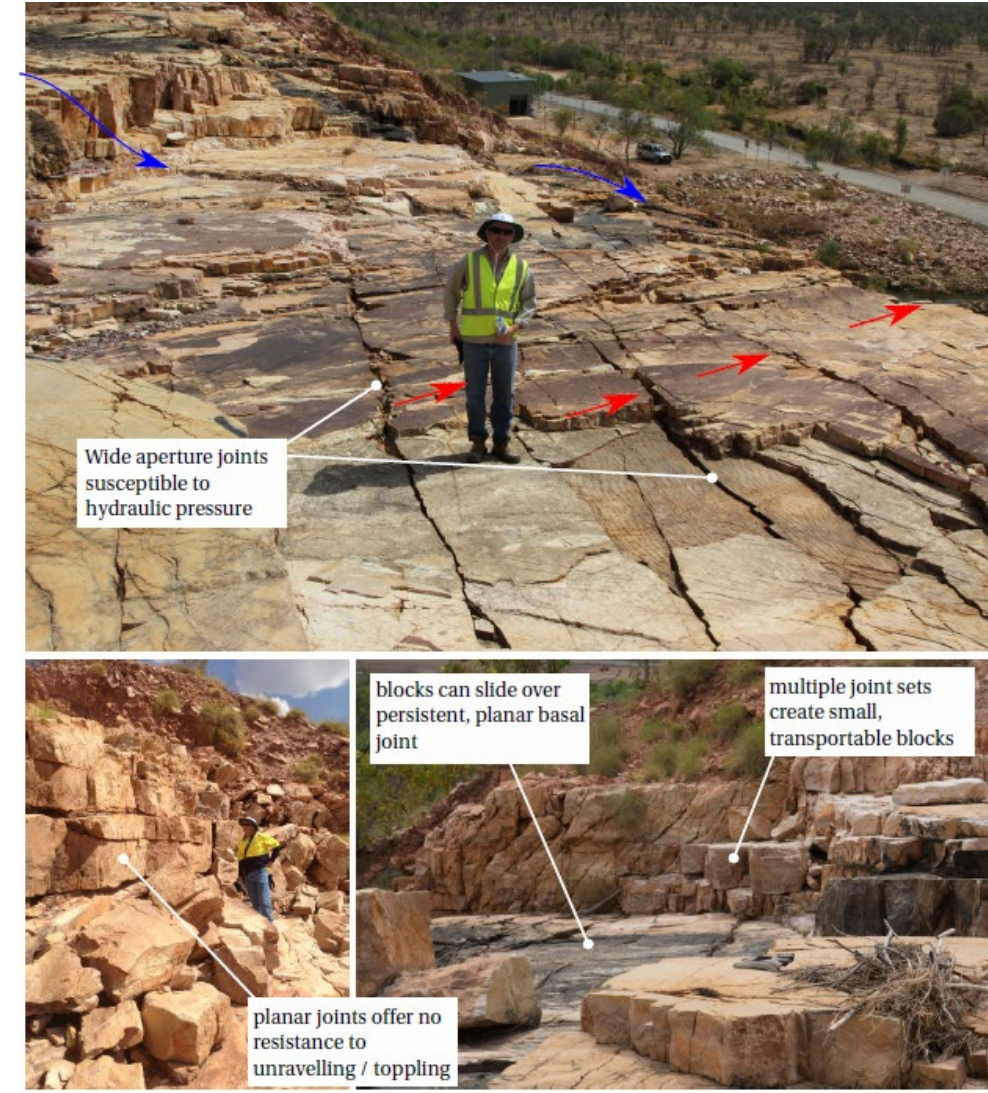
Figure 3.43 Moochalabra dam - sliding of jointed rock
